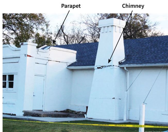
Masonry parapet separation.
